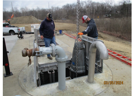
New Pumps at the New Lift Station 16
