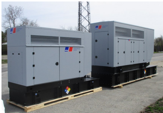
Generators for Lift Stations 11 & 14
