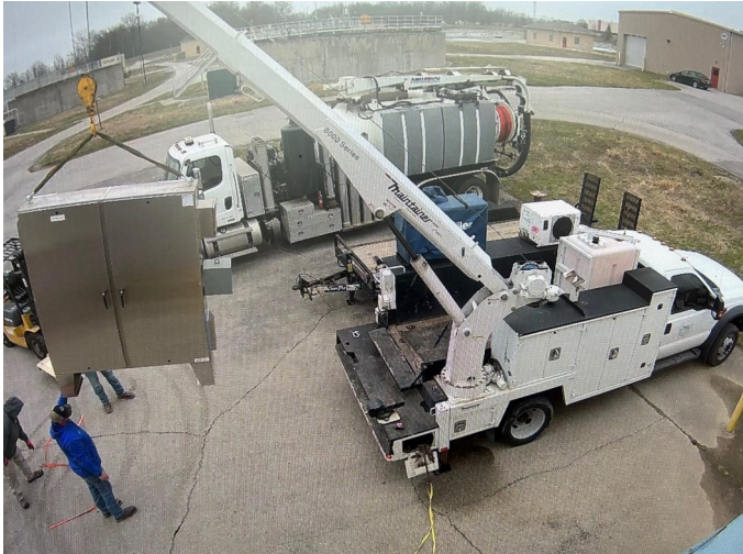
New Control Panel for Lift Station 14
