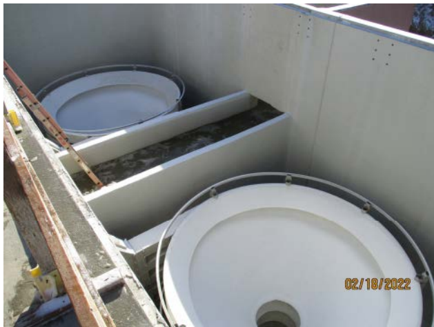
New Grit Removal Tanks
